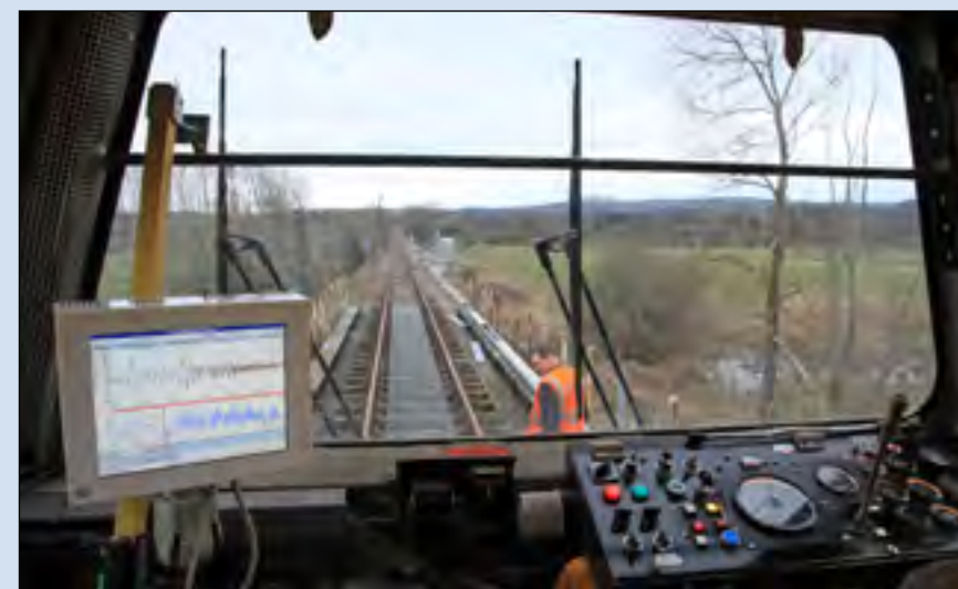
Some photos taken of tamping on the 'new section' of the Swanage Railway between Creech Bottom and Furzebrook.
