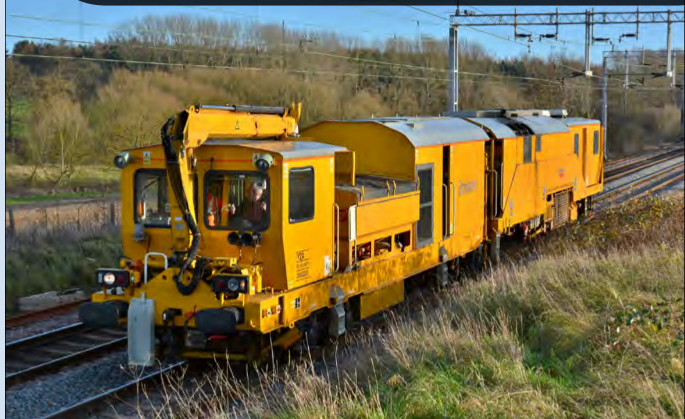
Stone Blower No. DR80205 heads north through Church Brampton on December 9th heading from Woking to Walsall Tamper Sidings. Geoff Barton
